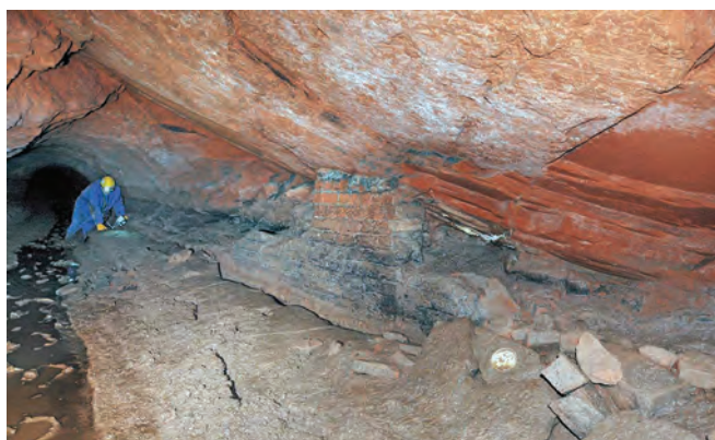
It was difficult to avoid sinking into the mud at the western end of the very wide section, where the roof has been reinforced with a brick pillar
